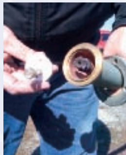
Damaged part on right, what it should look like on left
